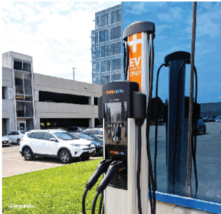
ChargePoint Level 2 EV charger at commercial building
